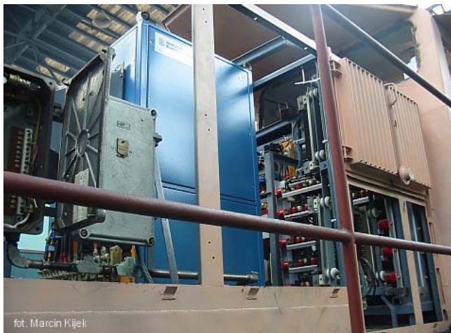
Figure 6, Chopper unit installed into E10 Locomotive
